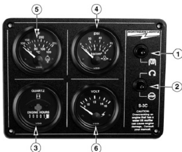
Figure 9: Series 3 Generator Control Panel
