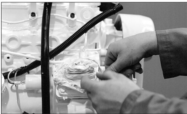
Figure 13: Cover lines, inlets and injection pump outlets.
